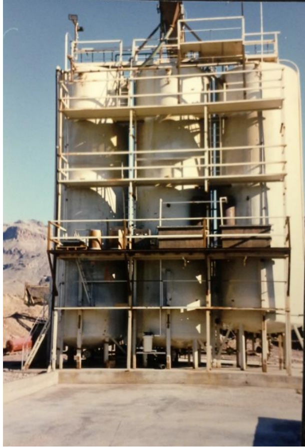
Figure 2.4 : 30,000 Gallon Cyanide Solution Tanks [1]
